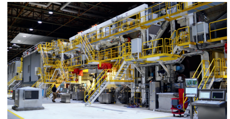
Paper Machine 1 at Somerset Mill
